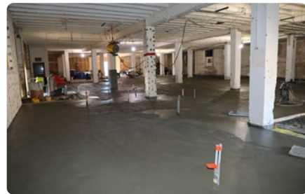
Interior view from the southeast corner of the Ford Building after floor leveling. Image courtesy of Jim Hanna
